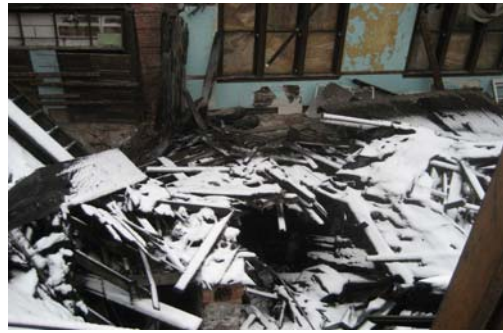
Gymnasium with collapsed roof and floor (Before)
