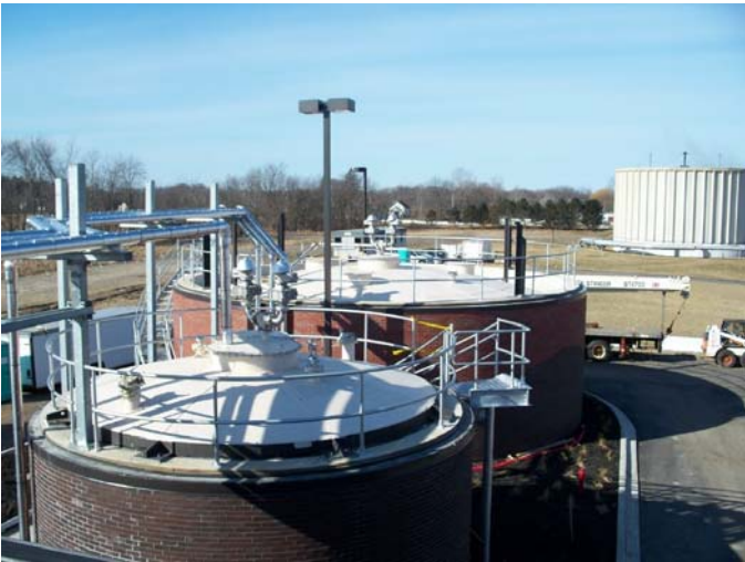
Photo 1: This photo shows a newly constructed thermophilic digester (foreground) and mesophilic digester (middle) at the Delhi Township WWTP. The gas piping will convey gas generated in the new digesters to the Digester Building, where it will be used to fire either the microturbines or the boiler. The existing nitrification tower is in the distant background.
