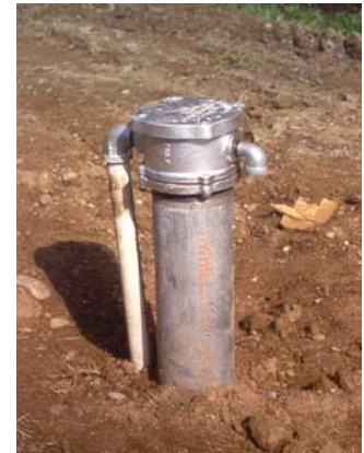
Typical Commercial/Industrial Well Head
