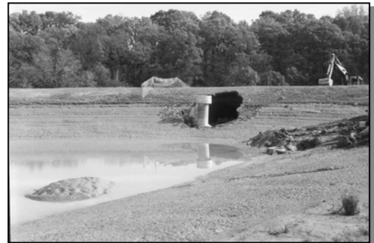
Structural failure of embankment
