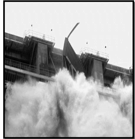
Structural Failure of Outlet Works
