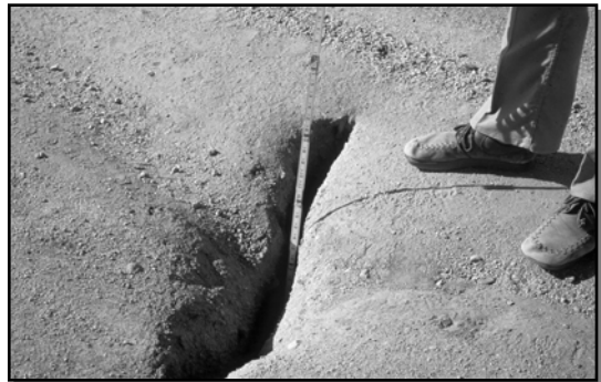
Large crack in the embankment
