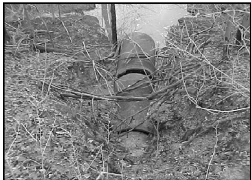
Severe outlet deterioration
