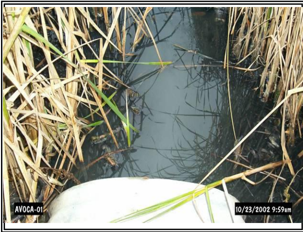
#211 County Drain Before: Prior to the project it was estimated that 15,000 gallons of raw sewage were entering the waterway each day.
