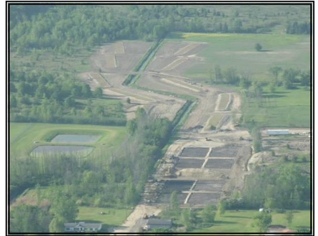
Aerial photo of the site of the wetland treatment system during construction.
