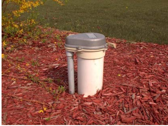
Typical wellhead for 5 inch PVC plastic well.
