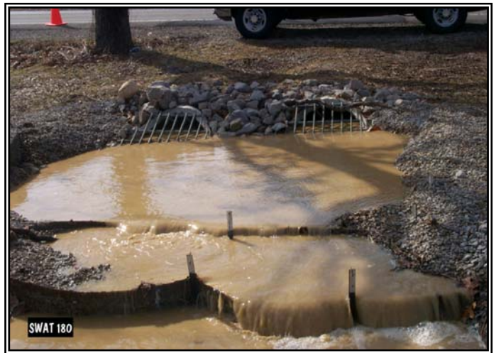
Runoff from construction sites with inadequate soil erosion control measures can affect water quality of lakes and streams and ponds.
