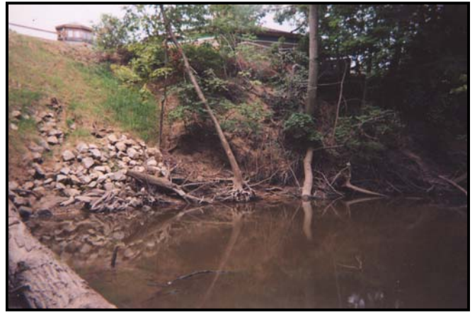
The stream bank near the nature center has extreme erosion potential. Attempts have been made to stabilize the bank with riprap and seeding.
