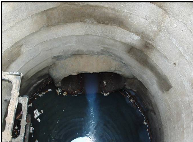
White discharge indicative of sewage discharge within the storm sewer
