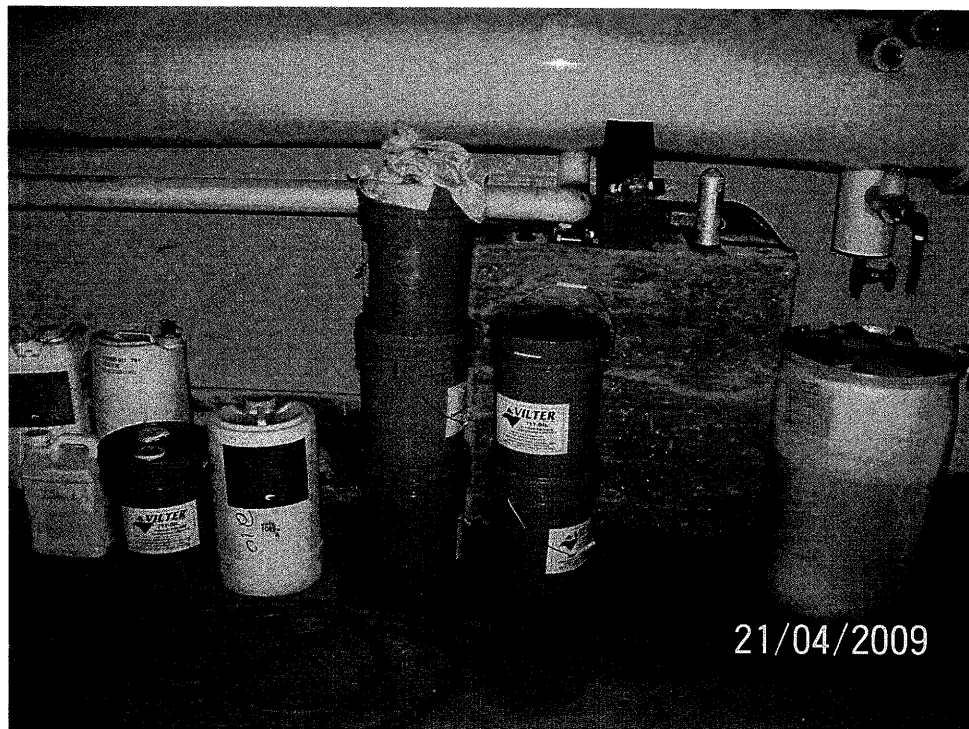
Photograph No. 18: View of the chemicals in the chiller (refrigerant) room of the Coliseum.
