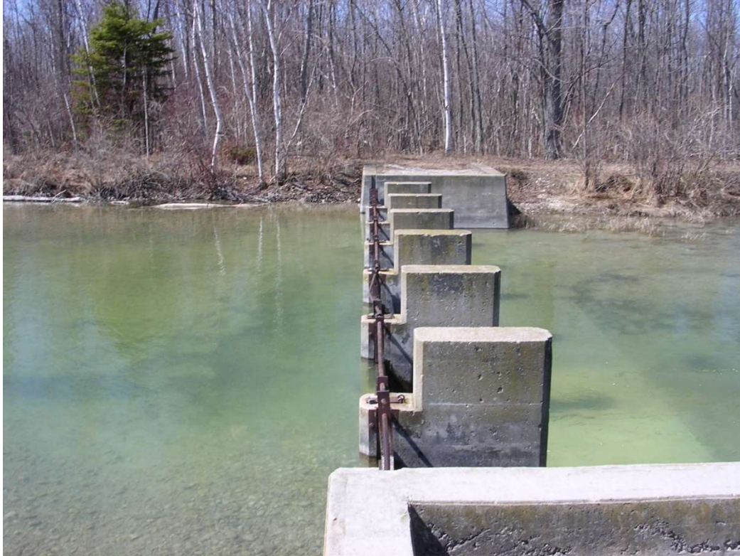
Photo 1.-Grand Lake water level control structure.
