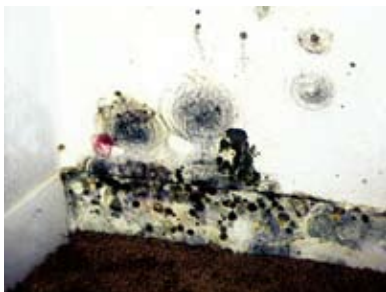
multi-colored mold growing on a wall
