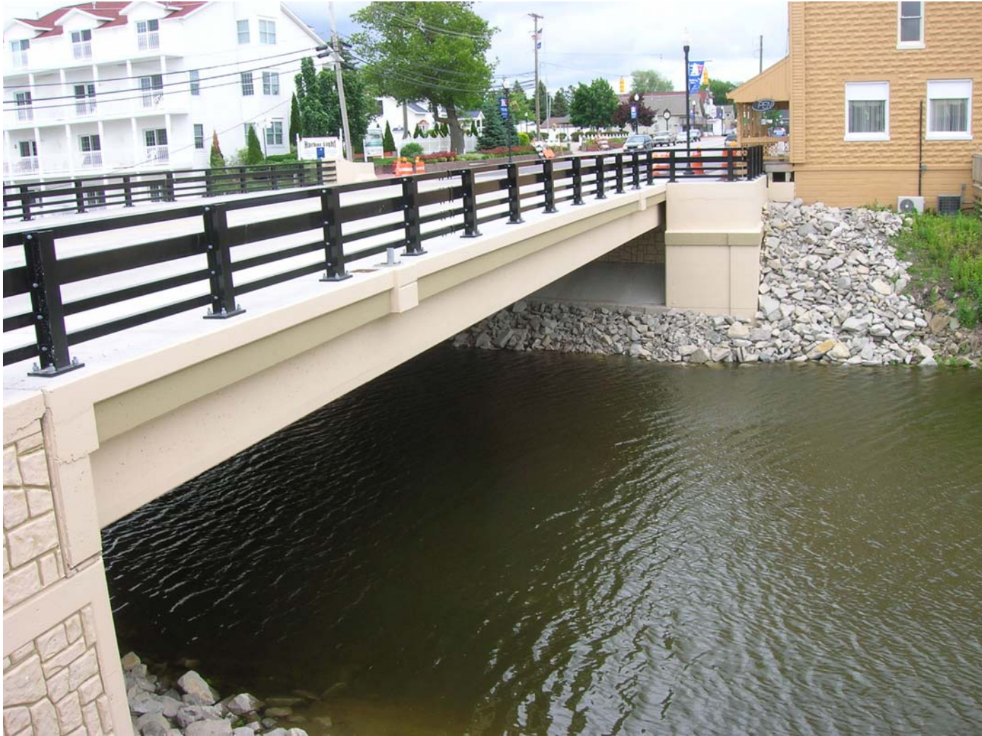
This photo of M-25 over the Pigeon River in the Village of Caseville shows what the railing on the bridge will look like.
