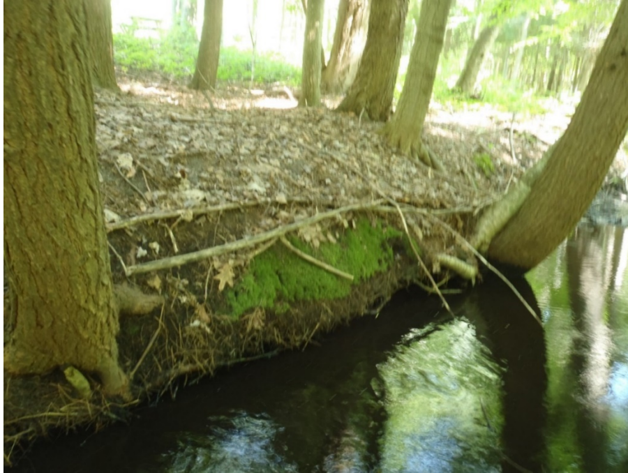
Figure 13. Eroded banks in the unnamed tributary to Little Platte Lake downstream of Saffron Road, Benzie County, Michigan.
