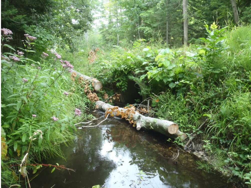
Figure 10. Unnamed tributary to Little Platte Lake. View of misaligned culvert upstream of Saffron Road, Benzie County, Michigan.
