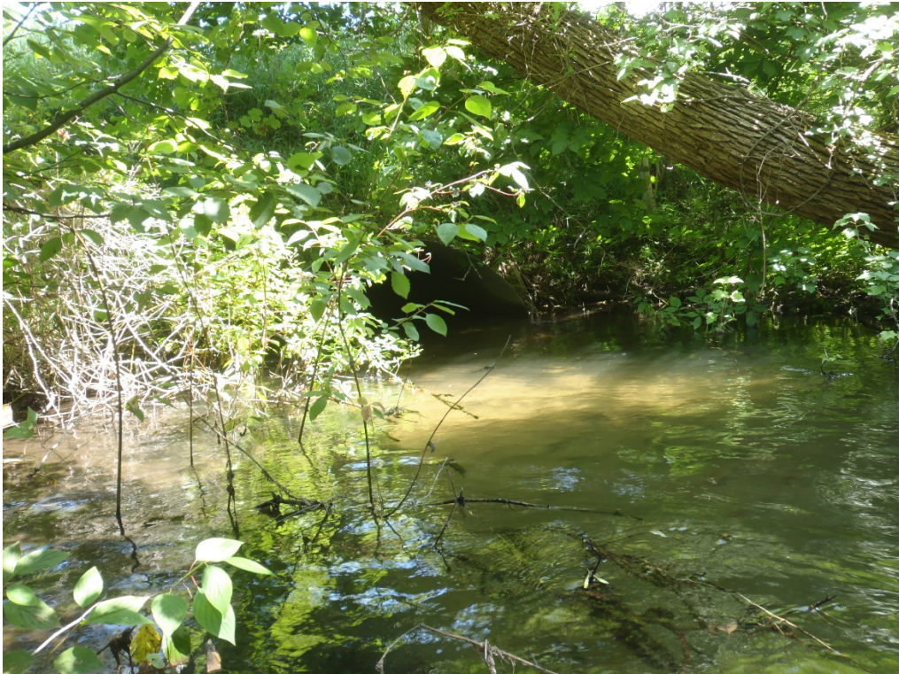
Figure 31. Undersized Culvert and widening of stream channel downstream of Gilbert Road, Bowens Creek, Manistee County, Michigan, August 2018.
