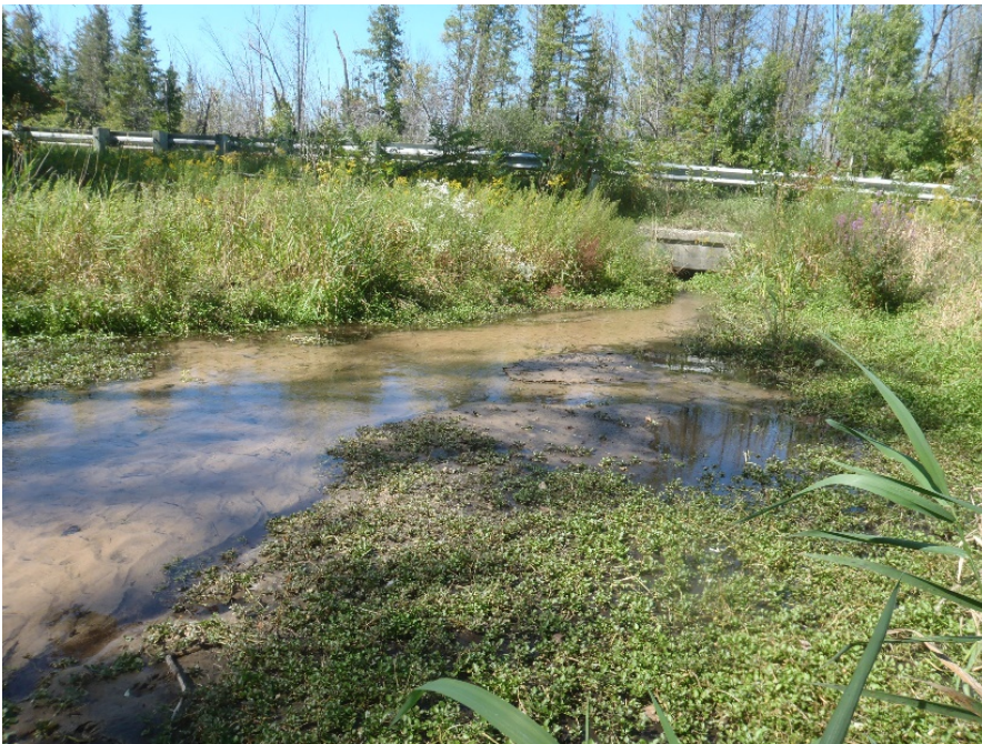
Figure 4. East branch unnamed tributary to Platte Lake Upstream of US-31. Note the large amount of sedimentation.
