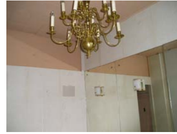
Picture right shows the women's powder room at the second floor level in fair condition.
