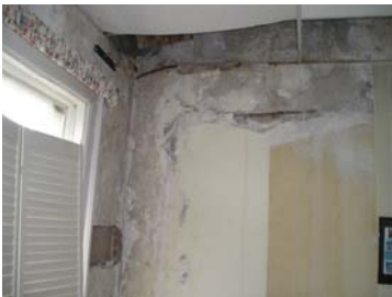
Picture left shows severe water damage to walls and ceiling in a lounge area at the second floor level.
