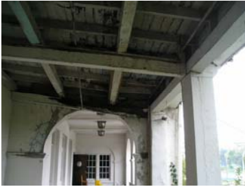
Picture left shows the entrance level terrace. The ceiling joists and soffits are in very poor condition.
