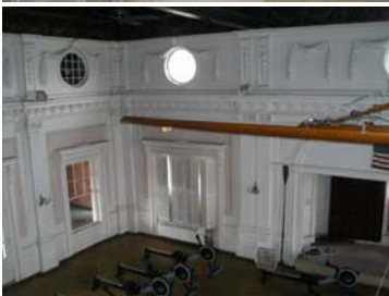
Picture left shows the ballroom from the mezzanine level over it. The space is in fair condition.
