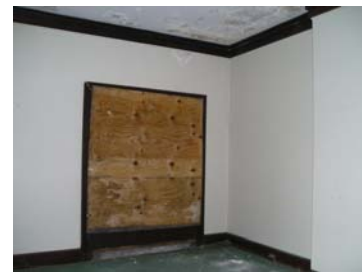
Picture right shows a boarded up window at the third floor window. The glazing is missing.
