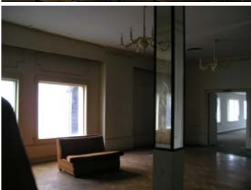
Picture left shows the River room which has wooden parquet flooring which is in fair condition.
