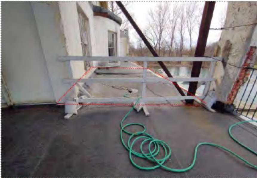
Photo No. 8 – Failed terrace slab viewed from topside.
