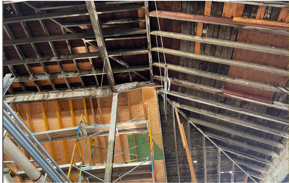
Roof is under- supported and needs replacement and reinforcement to stabilize roof.
