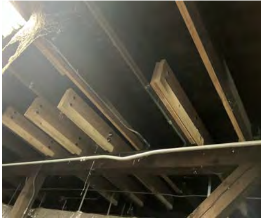
Structural reinforcement needed throughout the flat roof area and along the end beam on the west side of the roof. .
