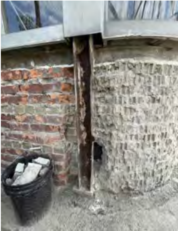
Deteriorated steel column was replaced.
