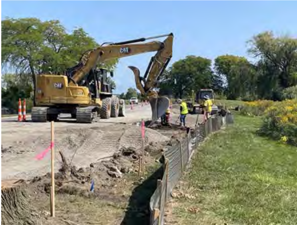
When complete, the road surface will accommodate the 2-way cycle track, 2 vehicular lanes and a multi-use bike path. ..
