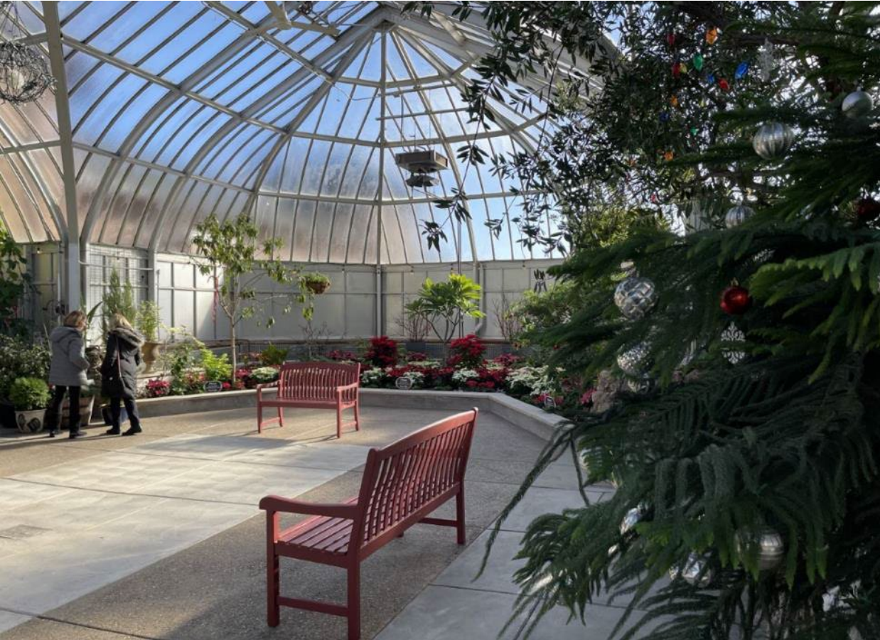
New floors and a new planter wall were installed in the showroom.
