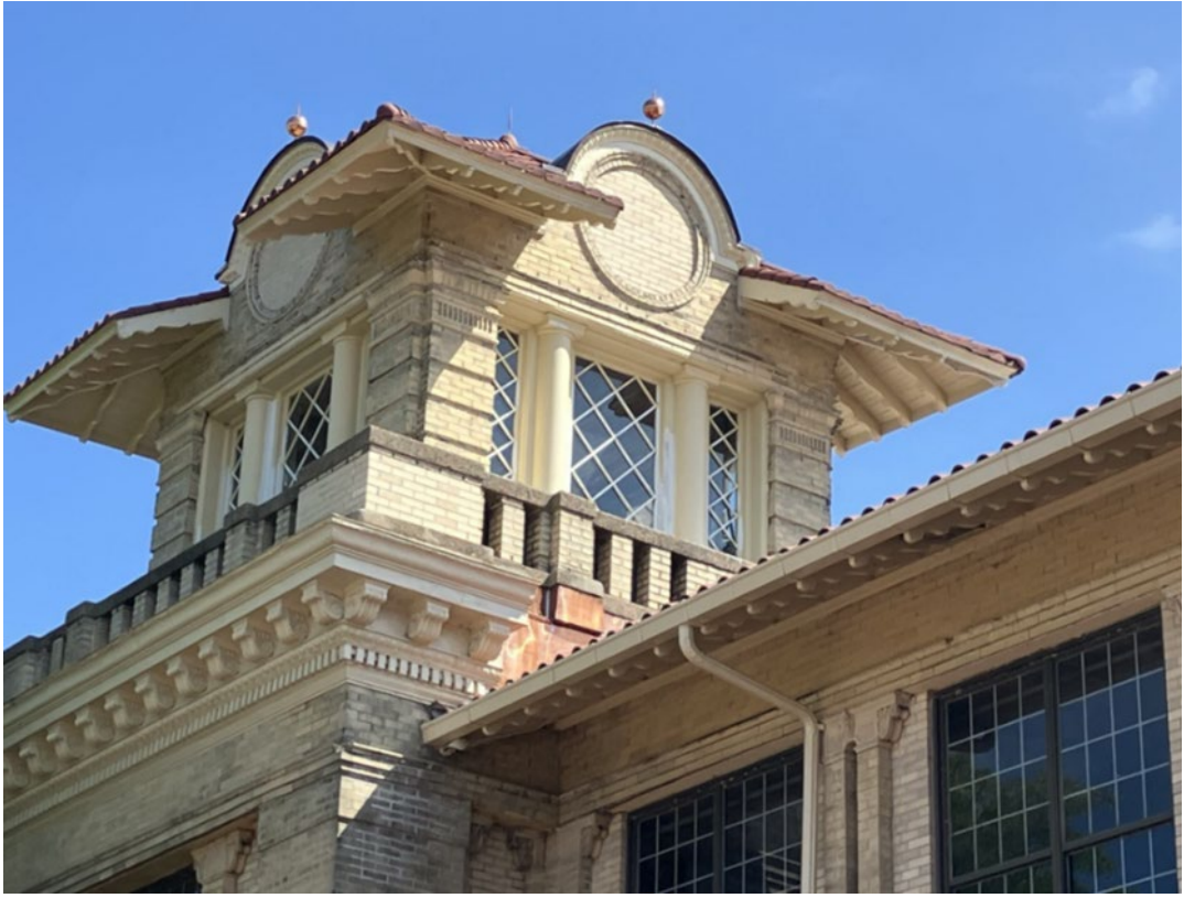
Complete replacement of clay tile roof, flat roof, skylight, drainage system, porch ceiling repairs, window repair, interior water damage repairs..
