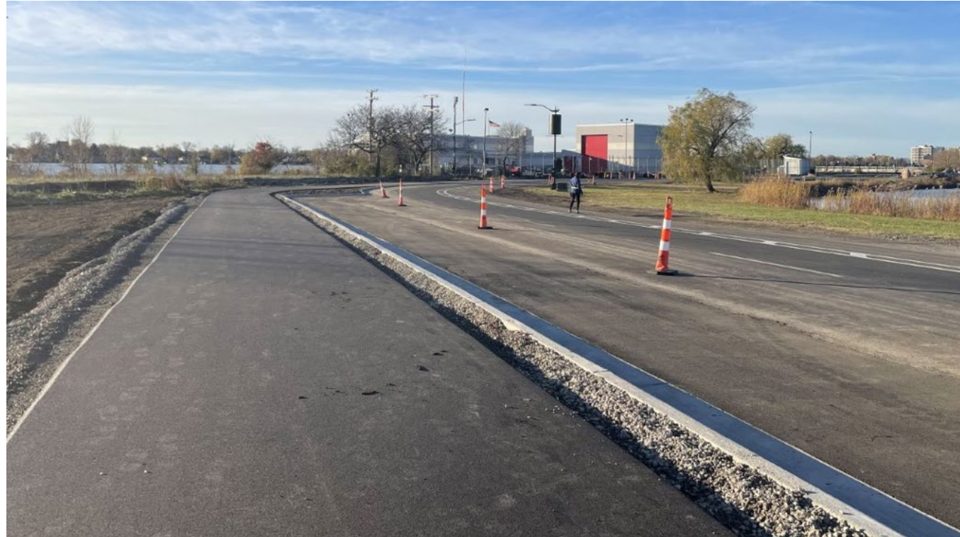
Wilson Trail Completed on south shoreline to the Lake Okonoka culvert for 2024.
