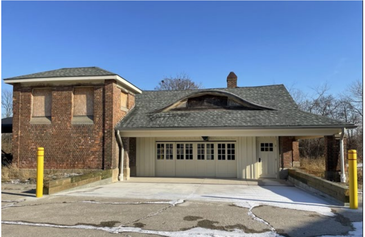
ADA access, site drainage and new doors installed in phase 2. Partnership between FRD and PRD.
