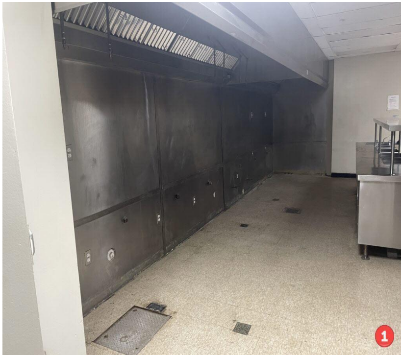
Figure 1. Wall repairs and gas lines capped earlier this year. Potential stove area with exhaust hood.
