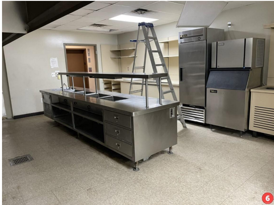
Figure 6. Food Preparation. Steam table, one-door refrigerator, ice machine.
