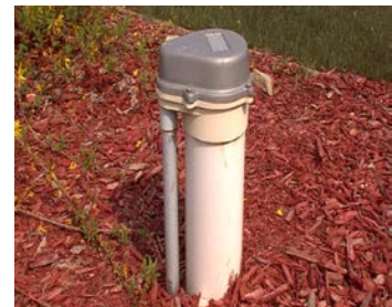
Typical Commercial/ Industrial Well Head
