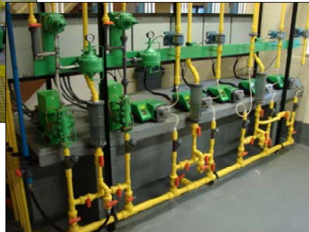
HOLLAND-SODIUM HYPOCHLORITE PUMPS
