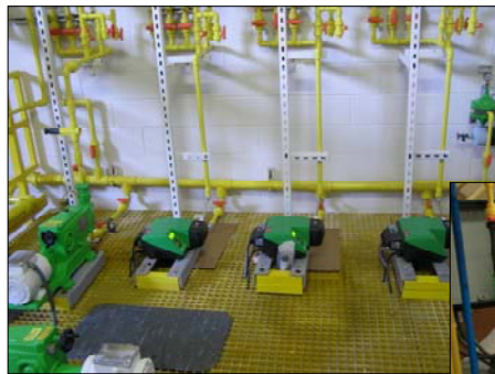
MUSKEGON-SODIUM HYPOCHLORITE PUMPS
