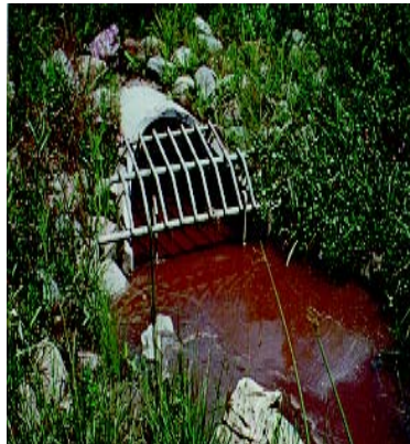
Typical Inlet Pipe
