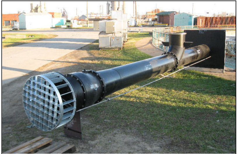
Each secondary clarifier requires a Return Activated Sludge Pump.
