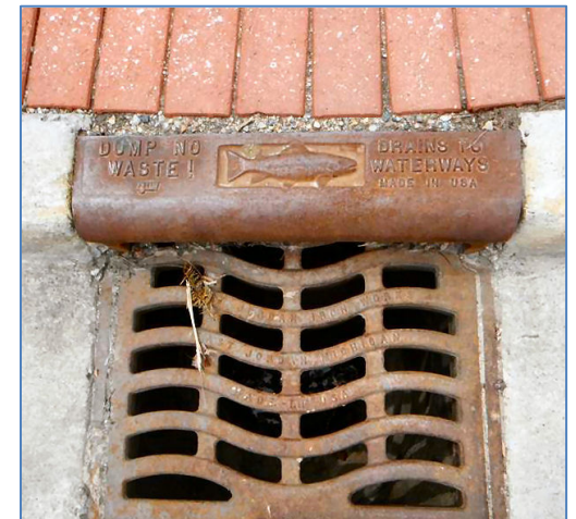
A catch basin grate casted with a reminder that stormwater drains to waterways.
