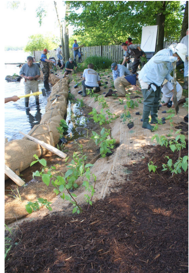
A trained crew installing a Demonstration Site. Photo by: Jane Herbert MSU Extension
