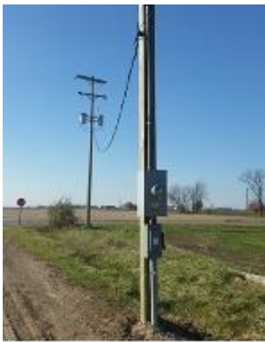
New Pole with new switch and meter socket
