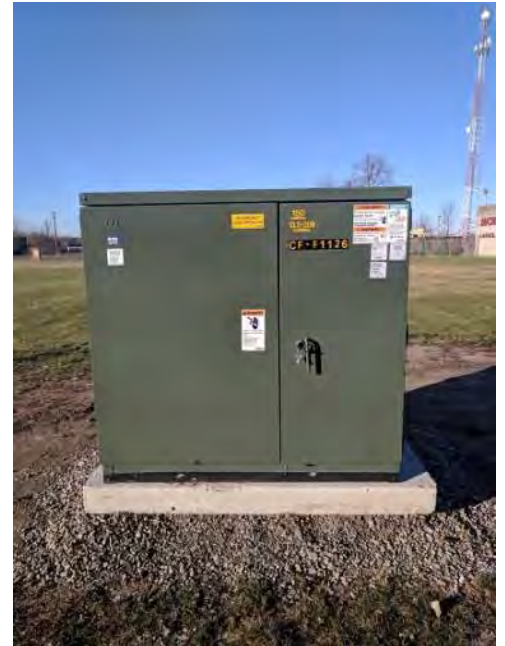
New Electrical Transformer
