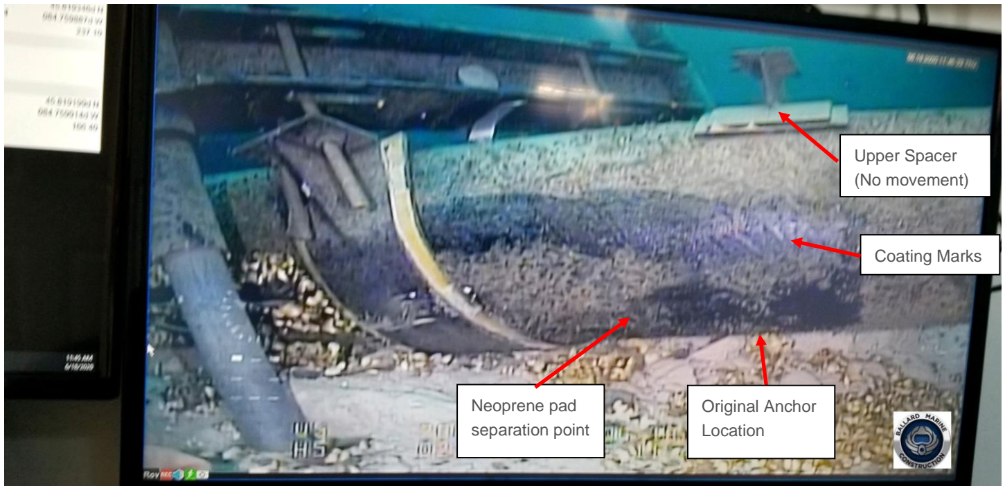
Figure 2: Displaced Anchor looking West
