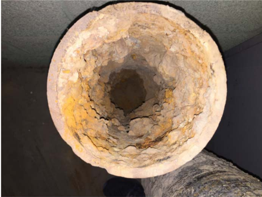
Figure 5. Tuberculation and scale thickness in an 8-inch cast iron pipe removed from Flint’s system.
