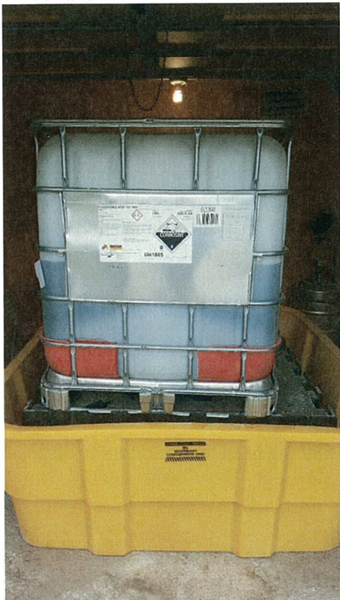
Figure 1: Existing Bulk Chemical Storage and Containment (phosphoric acid system shown in photo).
