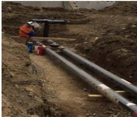
Heating / Hot Water loop piping installation showing proper excavation benching and sloping near Secondary Clarifier #s 1 & 2.
