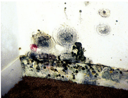
Mold growing on a wall.
