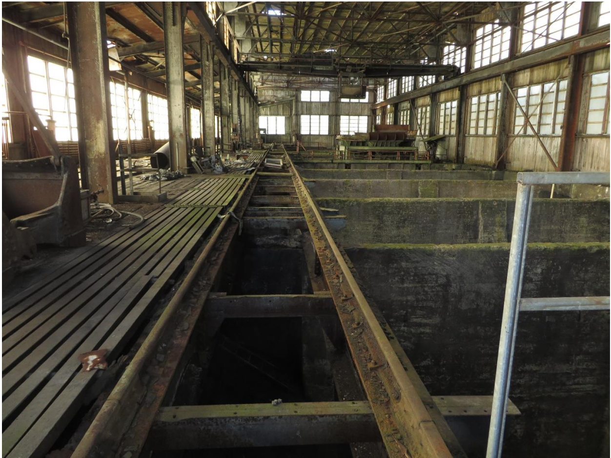
Photo 1: Mineral Building interior, looking southwest, with the bins (pits) on the right (MDEQ 2014)
