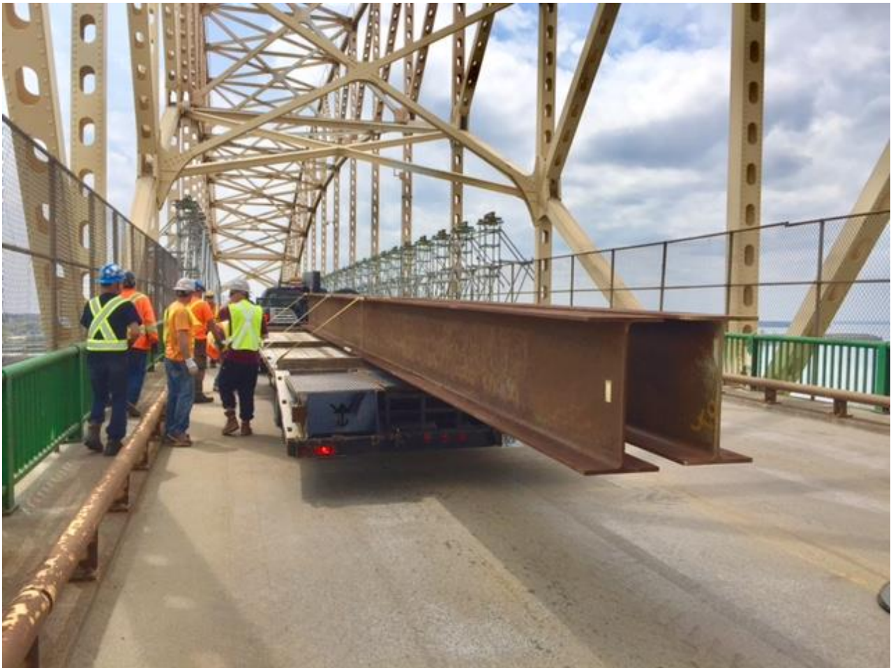
Caption: Workers install scaffolding and platforms on the Sault Ste. Marie International Bridge in preparation for this summer's $3.4 million Canadian arch painting project. (MDOT photo)
