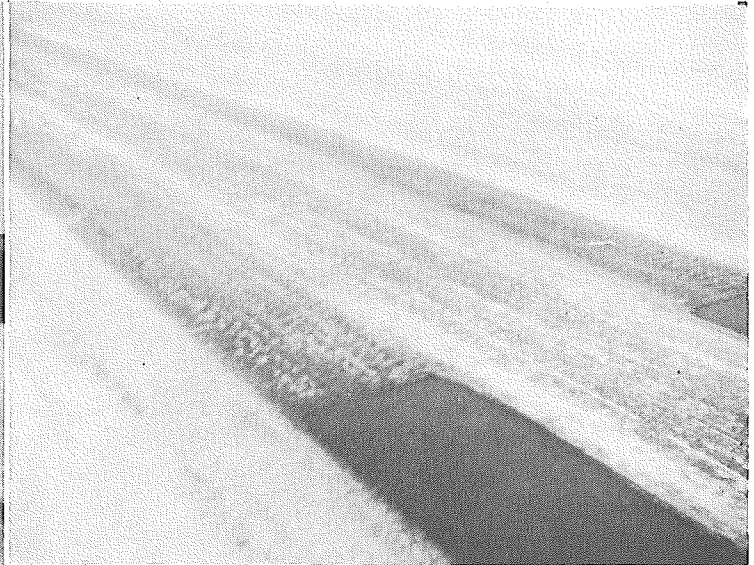
▲ FIGURE 2. BITUMINOUS SECTION ( 1 - 6 - 50 ) ICY CONDITION AT END OF SECTION
