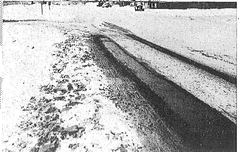
FIGURE 5. INSIDE TRACK ON BITUMINOUS SECTION PARTIALLY COVERED BY SLUSH FROM ADJACENT LANE. STORM 2/1/51
