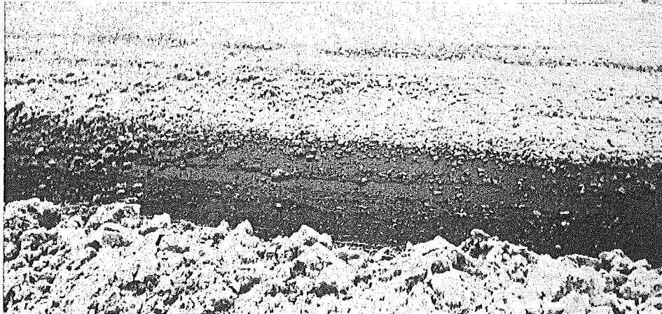
FIGURE 4. VIEW SHOWING INSIDE TRACK ON CONCRETE SECTION COVERED BY SLUSH FROM ADJACENT LANE. OUTSIDE TRACK IN FOREGROUND IS CLEAR. STORM 2/1/51
