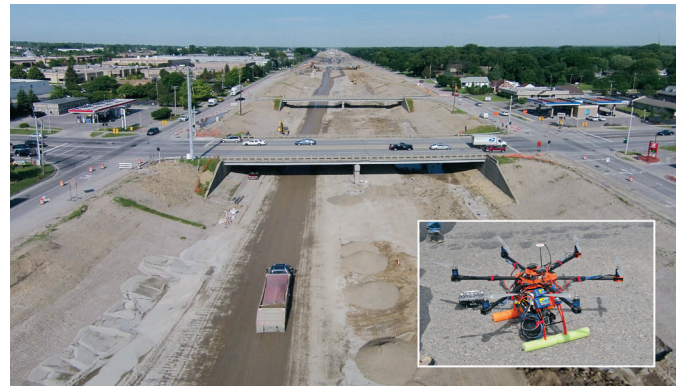
A Michigan-made unmanned hexacopter (inset) can gather aerial data quickly, like high-resolution imagery of this construction project on I-96 in Livonia.
