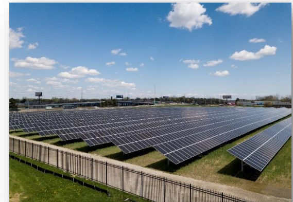
O'Shea Park Solar Array
