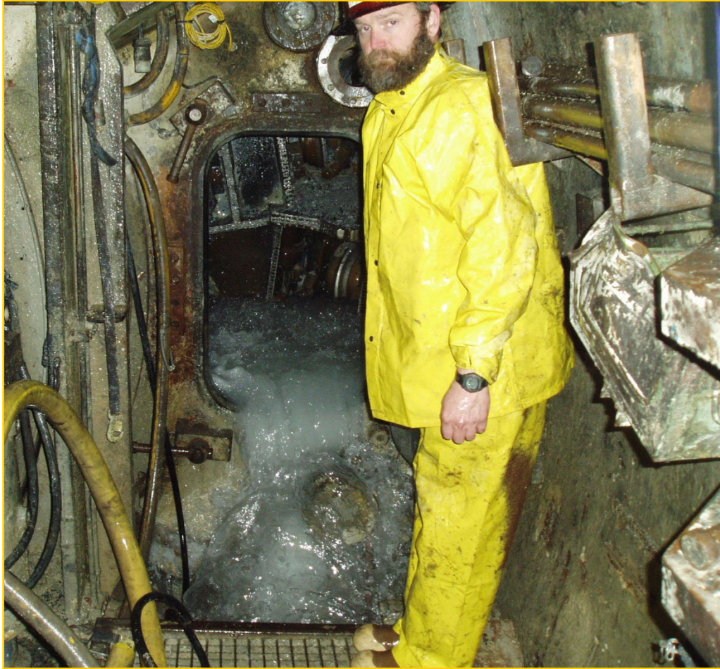
Figure 4 Water discharge (approximately 1,500 gpm) through a shielded TBM's open pressure bulkhead (cutter head beyond door opening) preventing maintenance/repair work within the TBM cutterhead chamber.
