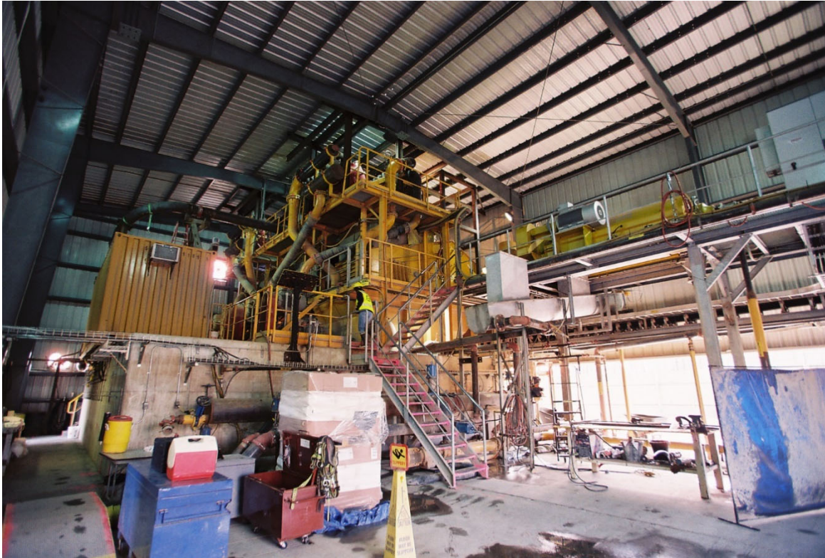
Figure 4. Inside Slurry Treatment Plant
