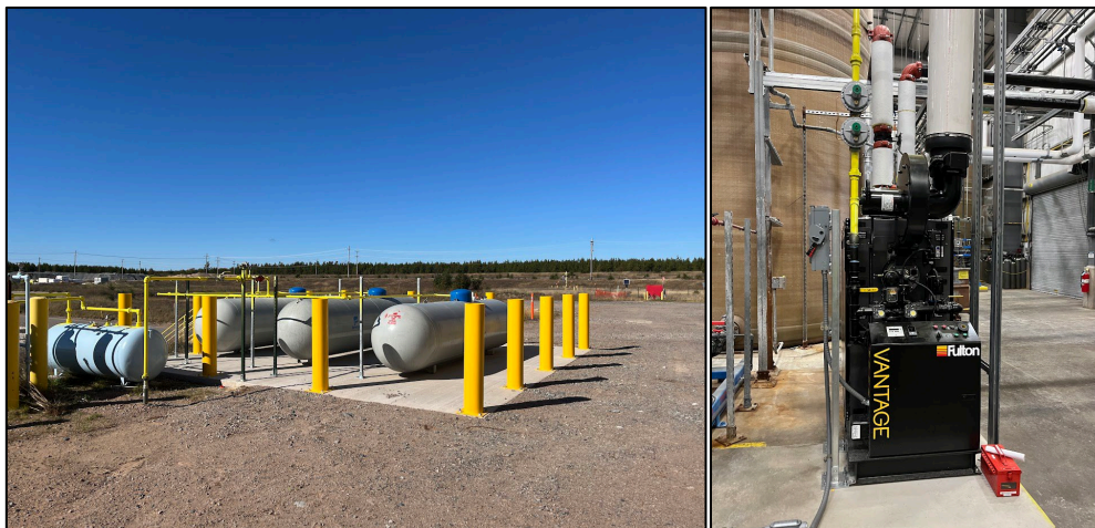
Figure 5 – New Propane Tanks at the WTP
