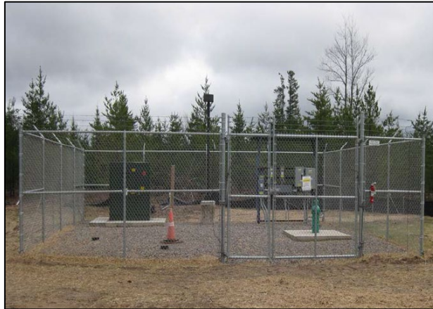
Figure 9 – Domestic Well at the Mine Site
