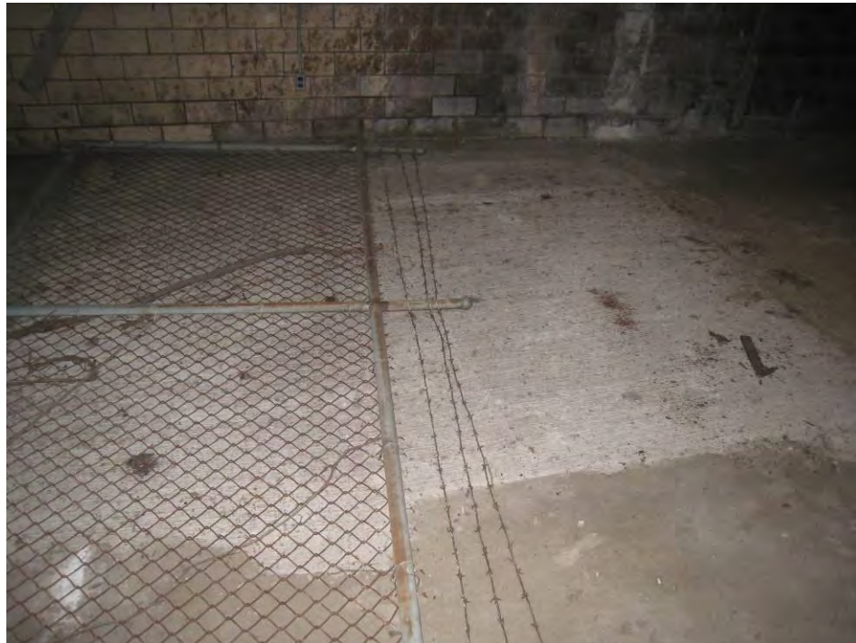
Photo 1 - View towards west of patched concrete floor at former ESCS location on 21 November 2011.
