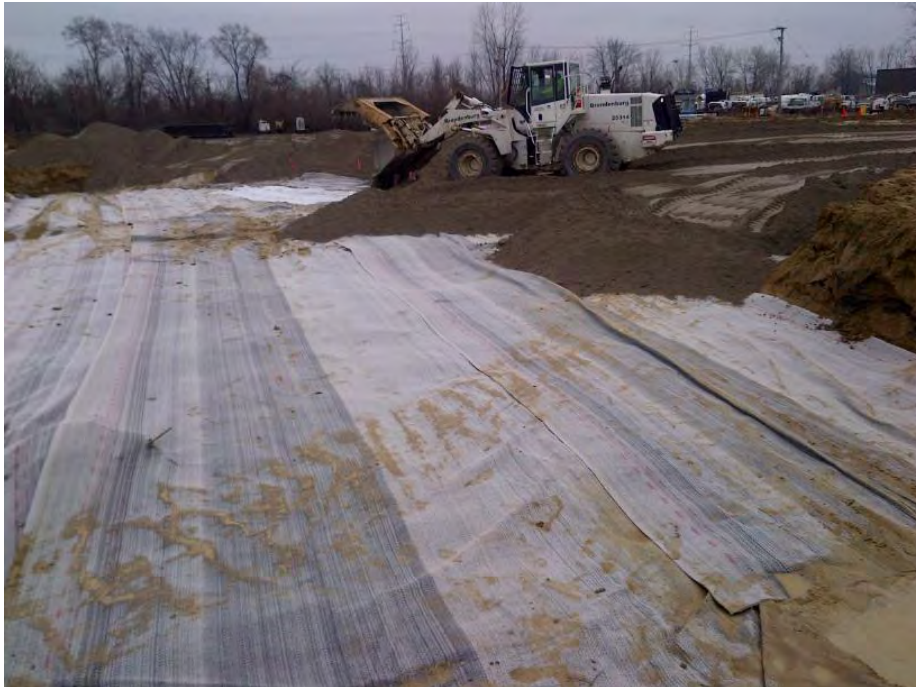
Photo 3 - Bentonite mat being installed in northern shop area excavation on 23 December 2014. Four feet of clean fill is being placed over the top of the mat. View is eastward.
