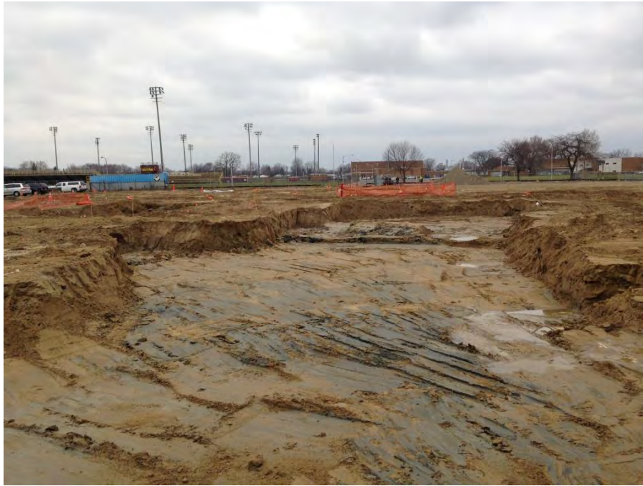
Photo 2 - View towards west of partially completed northern shop area excavation on 9 December 2014. Tan material is structural fill and gray material is underlying native clay. Note that perched water is practically non-existent within the excavation.
