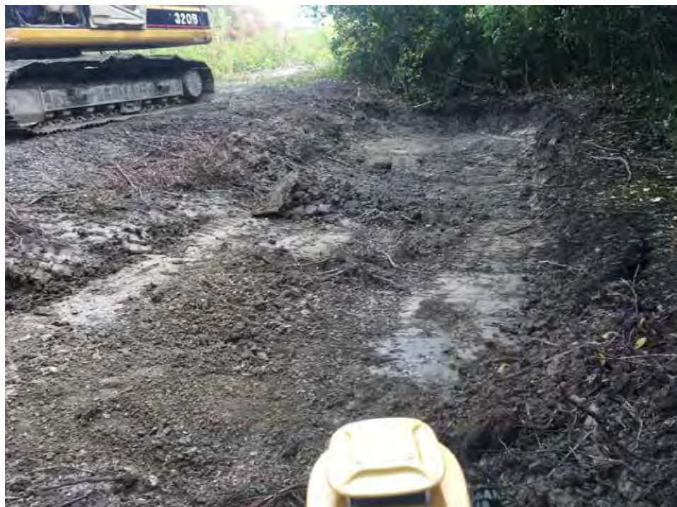
Photo 7 - View eastward towards ongoing Excavation #7 along south side of the rail spur on 20 September 2017.
