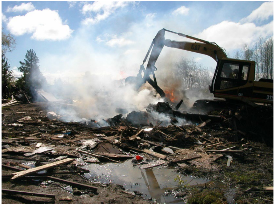
Illegal Burning of Demolition Waste
