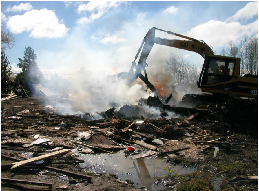
Illegal Burning of Demolition Waste
