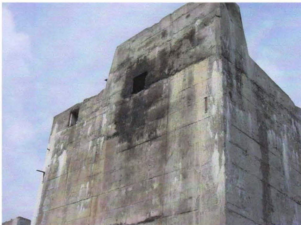
16. Photo shows staining on the side of concrete structure (looking north)
