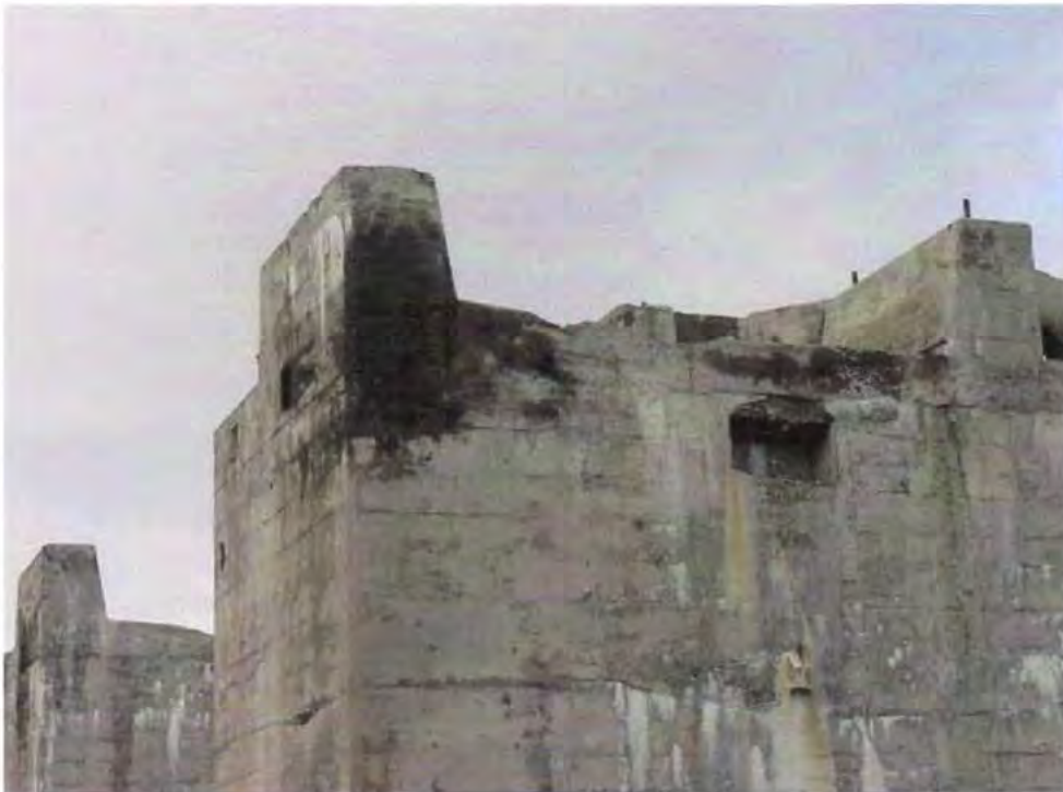
12. Photo shows staining on top of concrete structures (looking north)
