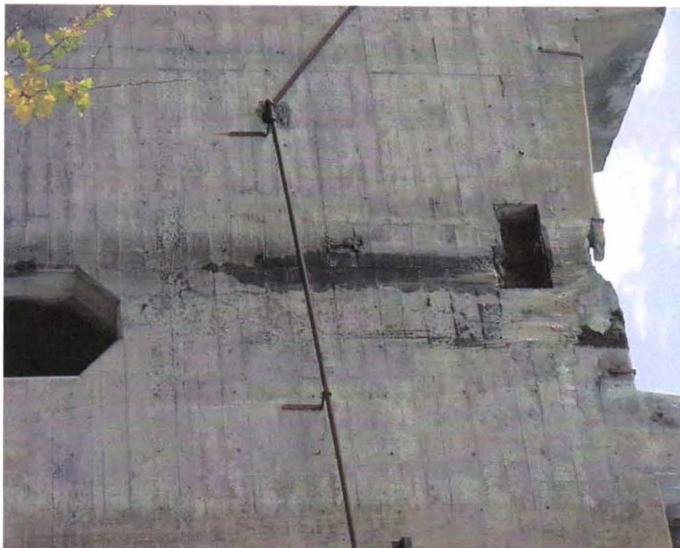
15. Photo shows staining on the side of concrete structure (looking north)
