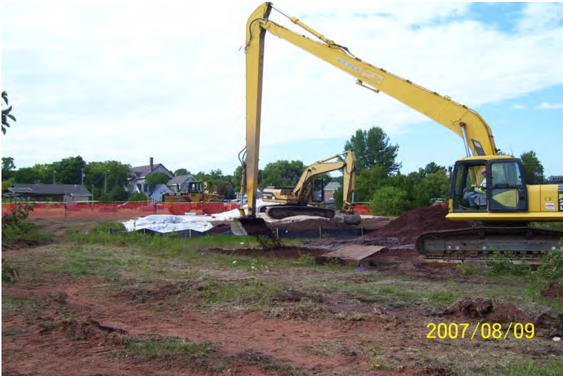
Site: Lake Linden ER Photo Number: 17 Direction: North Subject: Long-reach excavator in Area 1
