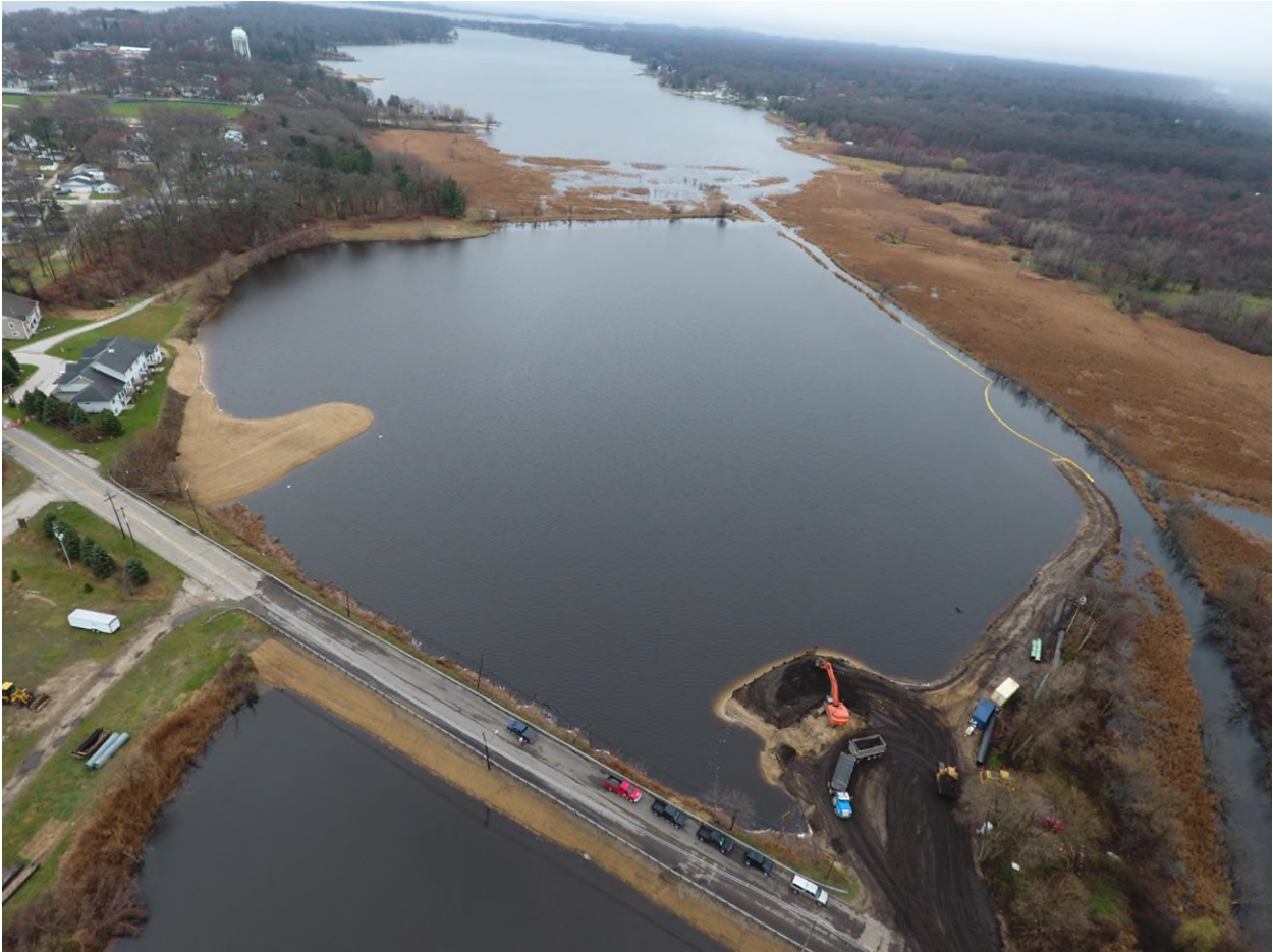
Figure 4. Earth work complete in the West Pond, including berm removal, looking west.
