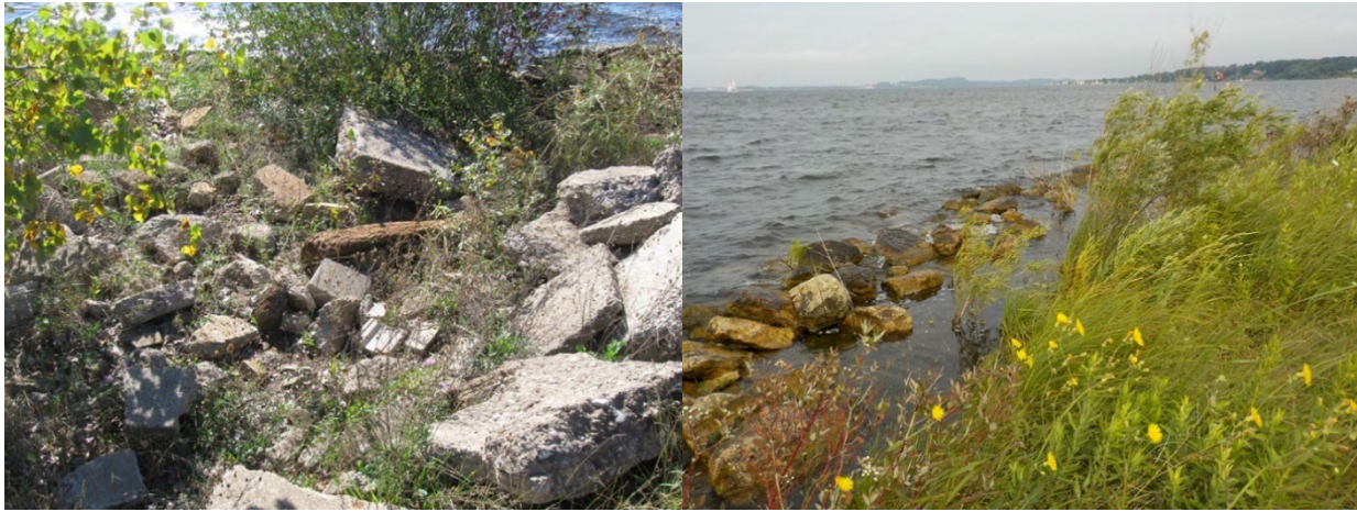
Figure 5. Center Point Bay Marina pre-restoration piles of rubble (left) and post-restoration facing north (right).
