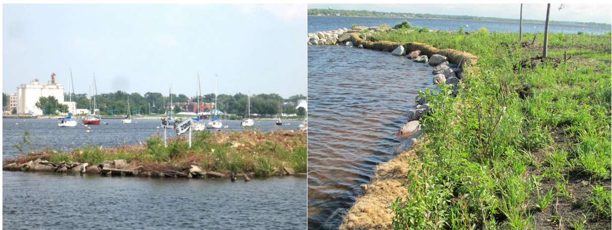
Figure 9. Hartshorn Peninsula before restoration with piles of debris (left) and after restoration (right).
